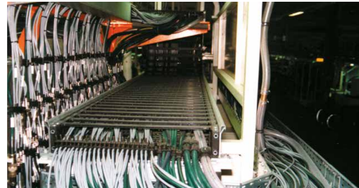
chainflex® CF5 and CF6 control cables (green) as well as CF211 measuring system cables (grey) in a screwing station of a car factory. e-chain®: E4/00 system with chainfix clip strain relief devices.
