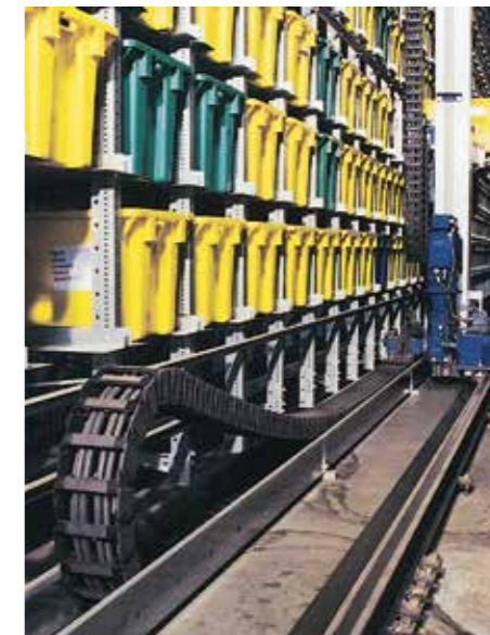
Automated storage/retrieval system with system E2 and chainflex® cables - travel lengths up to 80m and speed of v = 4.5\text{m/s}
