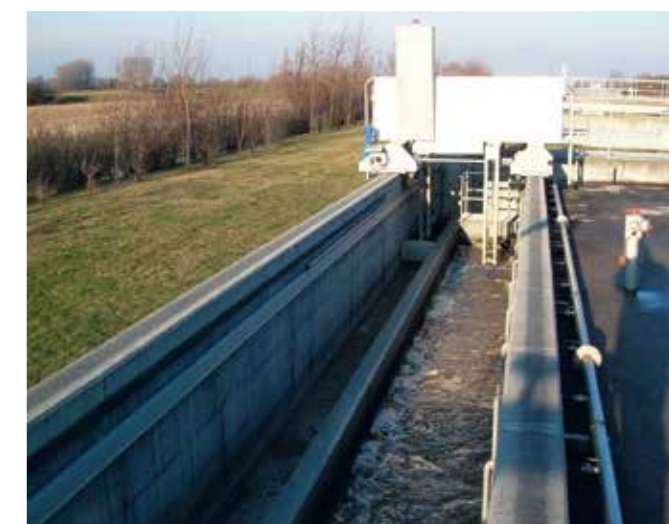
igus® micro flizz® in a sewage plant
