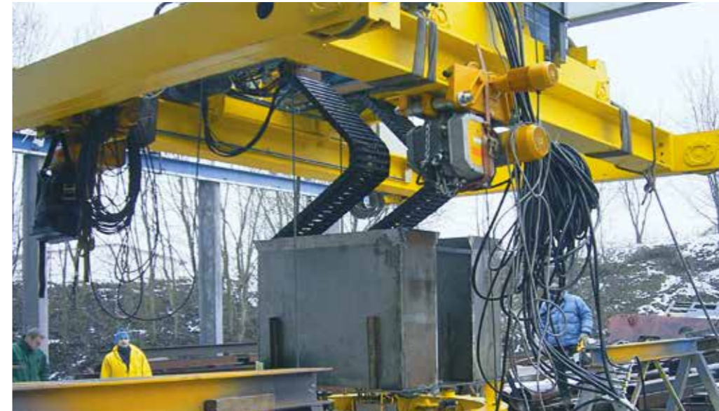
Zig-zag application: de-commissioning of a nuclear power station. About 14 m high steel containers are milled into small swarf for disposal
