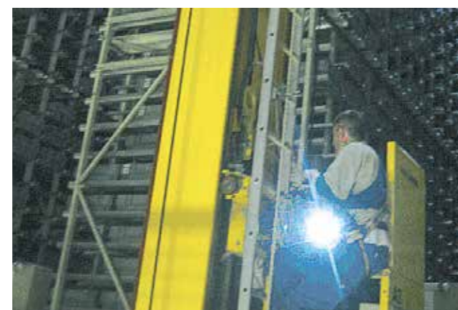
Short term, flexible installation dates even on weekends or at night - if you need immediate support or if the scheduled date has to be shifted. Simply give us a call and we will find a solution.
