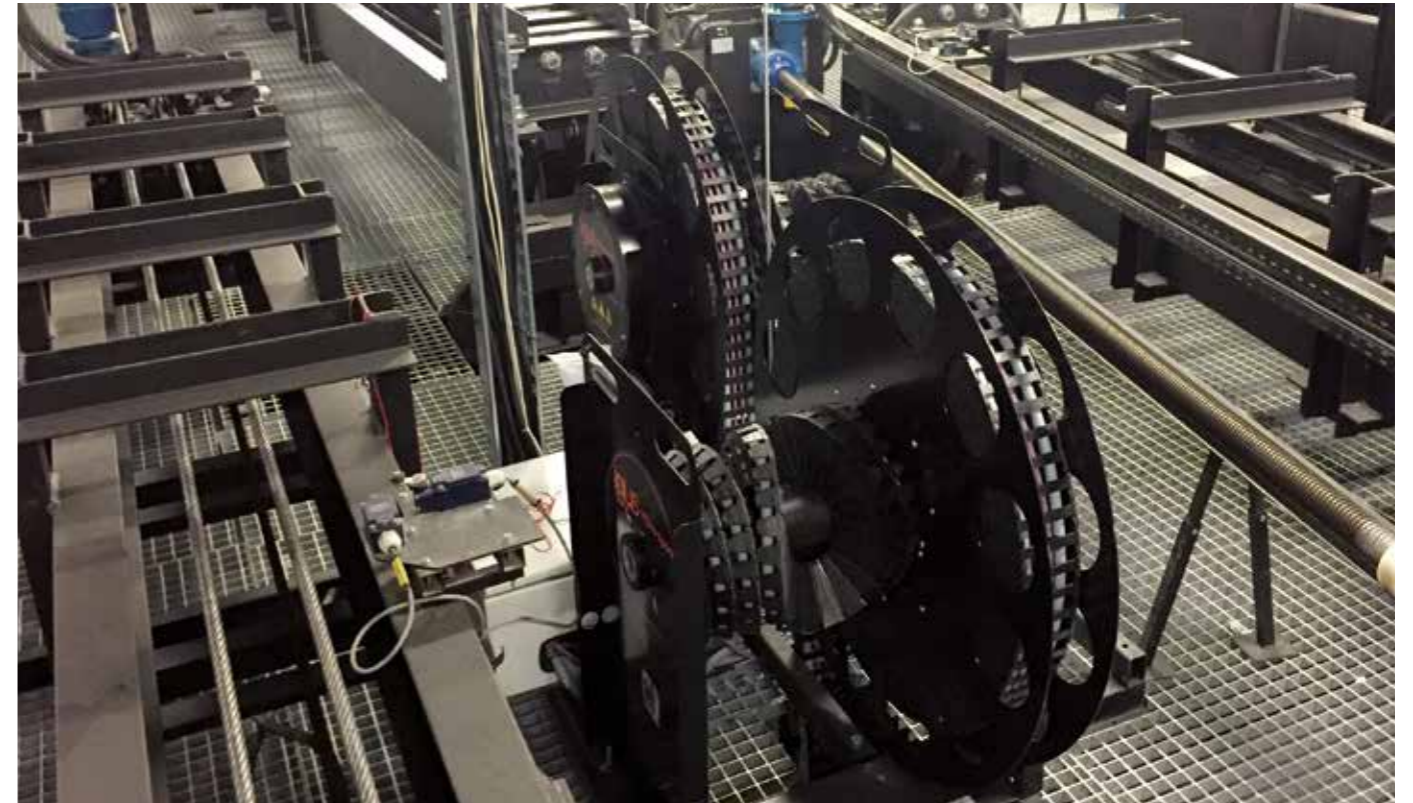
e-spool® - the solution for stage and theatre technology. Supplying energy, data and fluids without interruption. As shown here, at the Cultural and Congress Centre in Toruń (Poland). A total of ten igus® HD e-spool® systems have been installed
