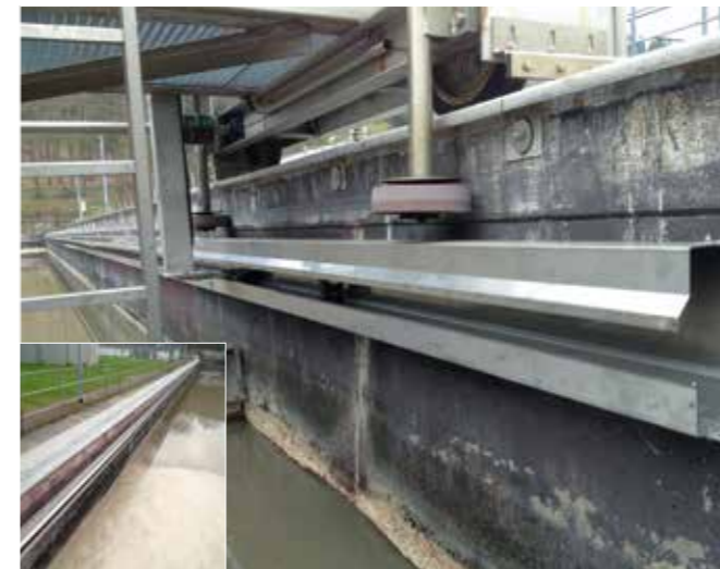
Longitudinal scraper, mounted in the basin, sewage treatment plant in Plauen, Germany - travel 53m
