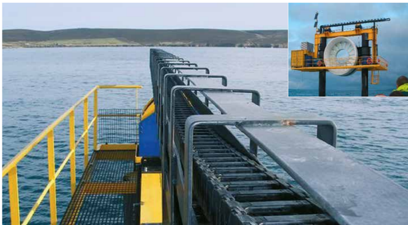
The maintenance-free series 4040HD protects the igus chainflex motor and signal cables during the lifting and lowering movements of this tidal turbine and protects them against the aggressive ambient conditions. 20m vertical movement above and below water
