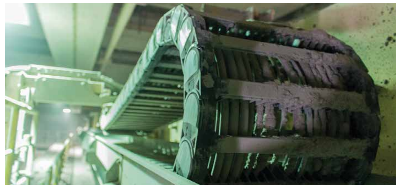
A heavily dust-filled, warm and humid climate pose a great challenge to the components used in this waste bunker
