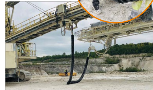
The e-loop® is used in the bucket wheel excavator of the company Holcim (Germany) GmbH. The modular system made of high-performance polymer always enables a defined bend radius and easily copes with vibration and impact.
