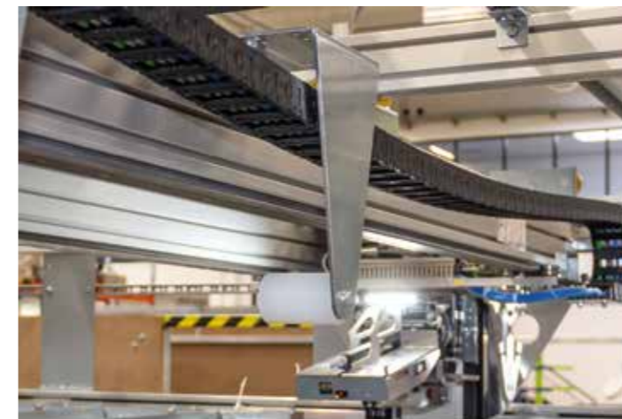
chainflex® cables (e.g. CF211) and igus® e-chains® (E065 series) in a pharmacy picking systems
