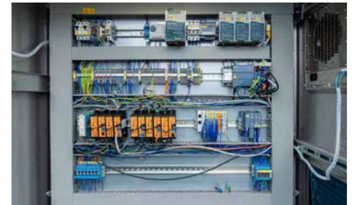
Switch cabinet with smart plastics modules
