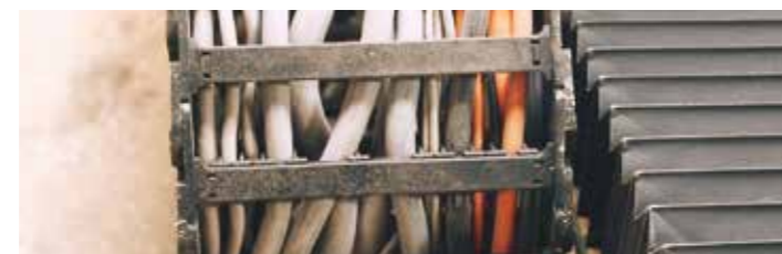
Corkscrewing: an effect of improper cable and hose placement in an e-chain®
